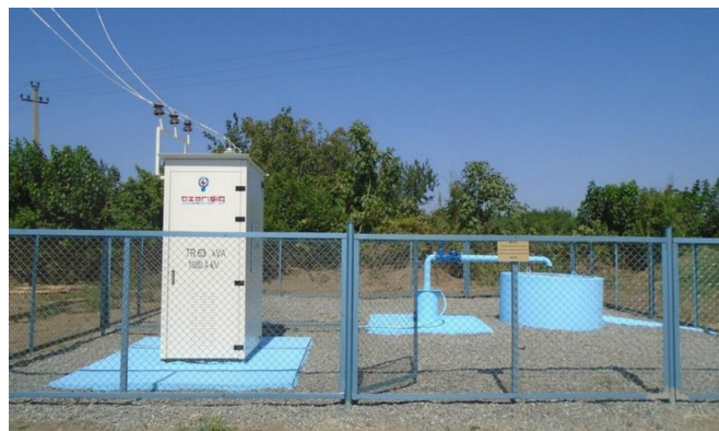
Fig. 3. Artesian wells surface equipment
